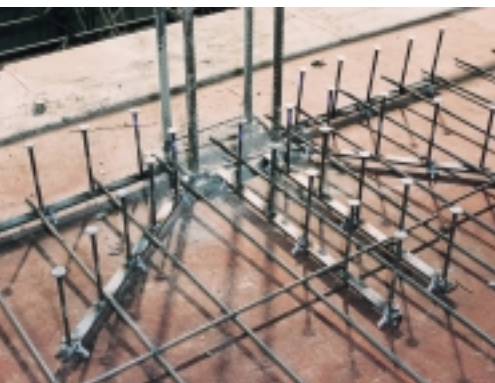
Figure 5: Stud rails at Cardington
